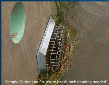
Sample Outlet and Structure (trash rack cleaning needed)
