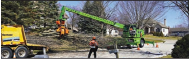
A specialized telehandler being used to quickly move material into a large chipper.
